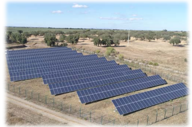
Example of a 2MW community-scale solar PV project
