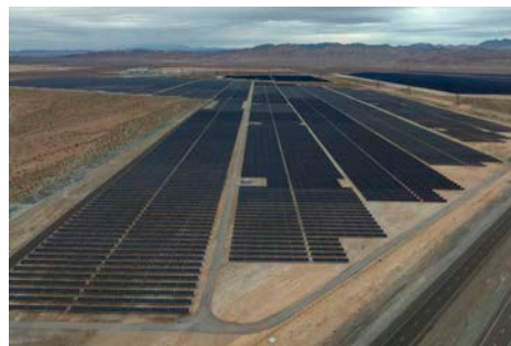
100MW utility-scale solar PV facility north of Las Vegas
